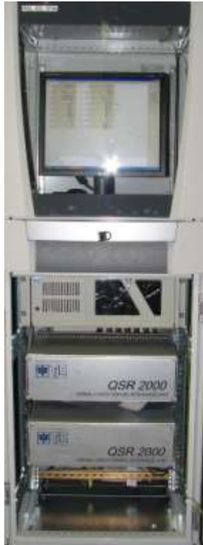
Fig 1: Rack Mounted Advanced Monitoring System
