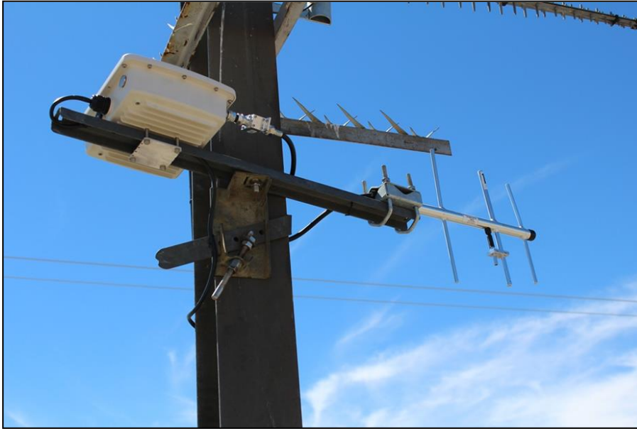
Fig. 3. Example of radio site installation
