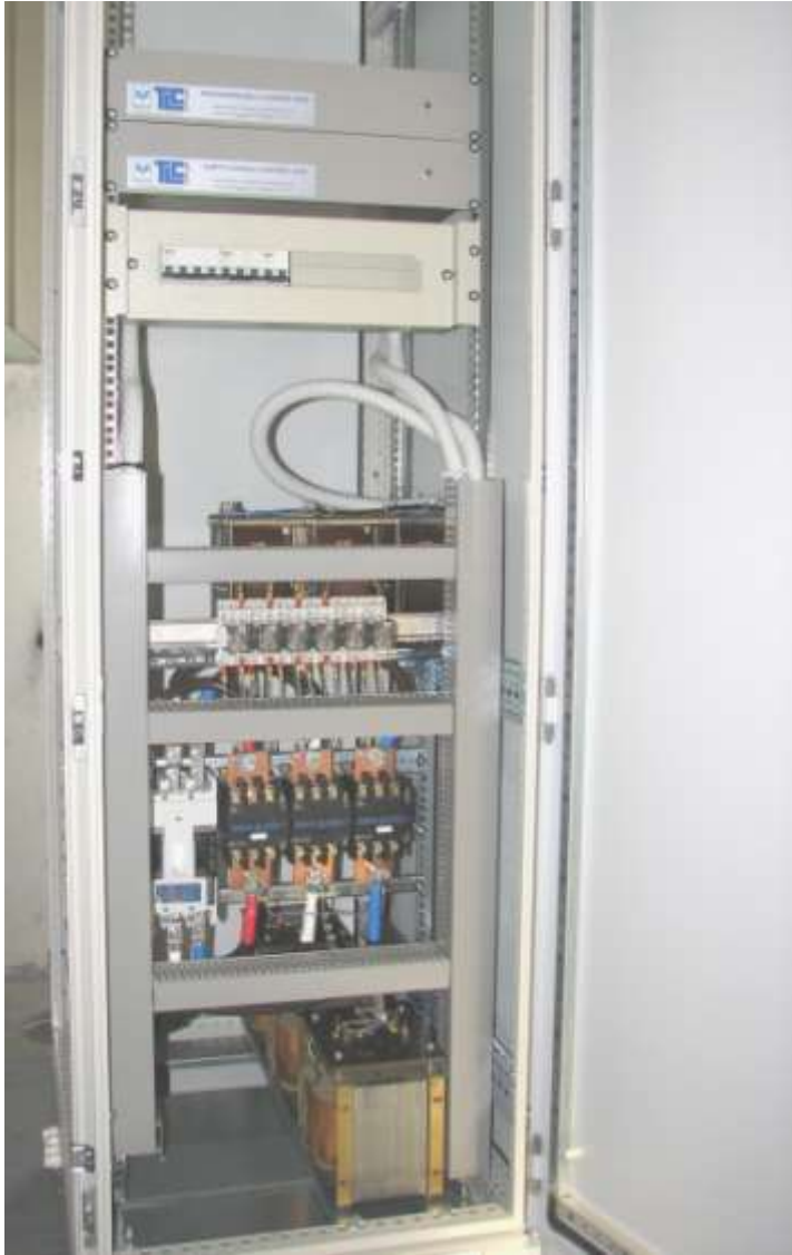
Fig. 14: Earth Leakage Test Unit Equipment
