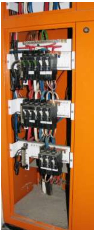
Emergency Supply Panel
