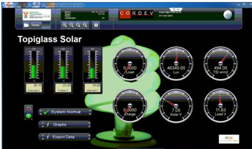
Figure 11. BMS Data Display
